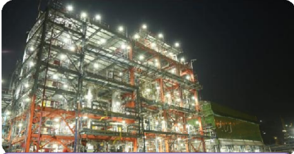
35 TMTPA INDAdapt G Plant at Guwahati Refinery
